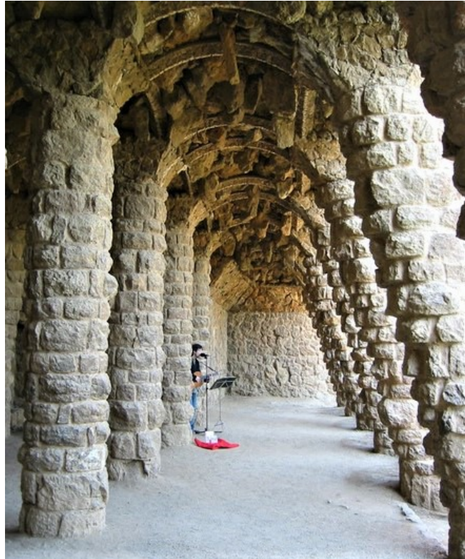
Columns supporting the vault carry the weight of the roadway viaduct in Parc Güell – Author, Usuario Rapomon, Wikimedia
